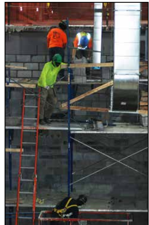
Workmen completing a new second floor area in the former drill shed of the New York State Armory in Jamaica, Queens on March 7, 2023. The $100 million renovation of the armory, which takes up a city block, is due to be finished by the summer of 2024.
