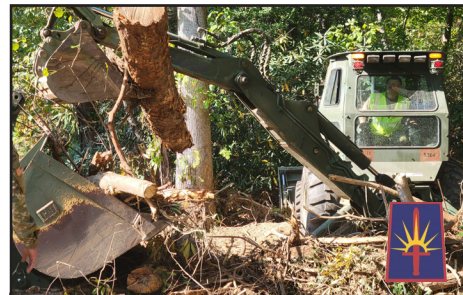
Engineers assigned to the 204th Engineer Battalion work to clear downed trees in the vicinity of Old Fort, N.C. on Oct. 13, 2024. The battalion deployed 20 Soldiers with engineer equipment as part of a 47-Soldier contingent which deployed to help the North Carolina National Guard cope with damage caused by Hurricane Helene. Courtesy photo.
