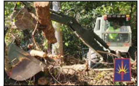
Engineers assigned to the 204th Engineer Battalion work to clear downed trees in the vicinity of Old Fort, N.C. on Oct. 13, 2024. The battalion deployed 20 Soldiers with engineer equipment as part of a 47-Soldier contingent which deployed to help the North Carolina National Guard cope with damage caused by Hurricane Helene. Courtesy photo.
