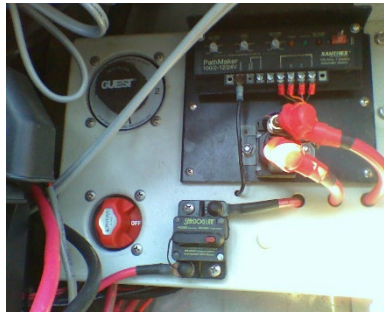
(Battery Isolator – Starboard Side Aft)
