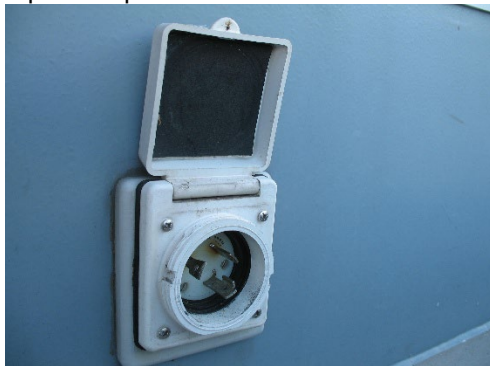
Shore Power Inlet
