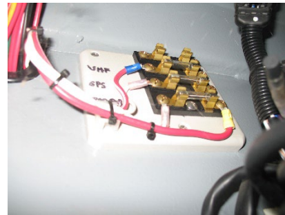
(Fuse Panel Under Helm Console)
