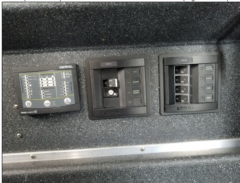
(Electrical switch panel)
